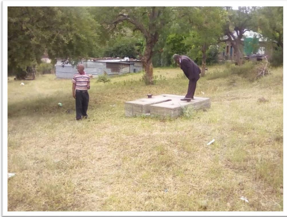
Figure 10: Dilapidated Borehole at Moeng Section (seen here is Ward Councillor and Nduna)
