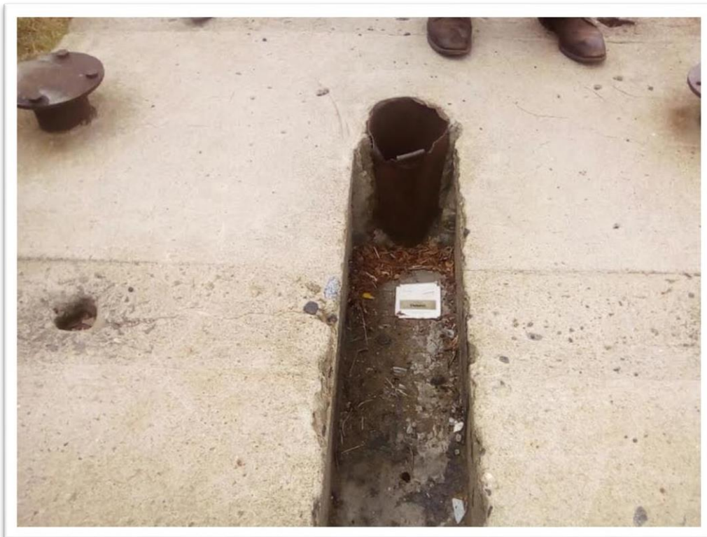
Figure 6: Dilapidated borehole drilled by Samancor with rubble stuck into borehole
