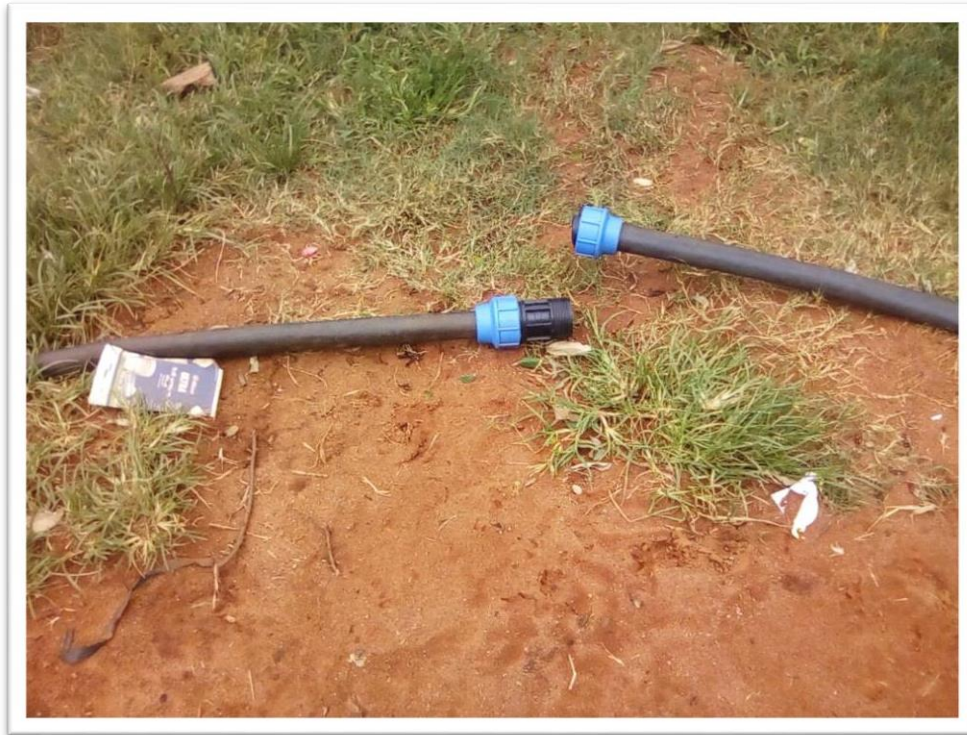
Figure 12: Damaged coupling at Kampeng Section
