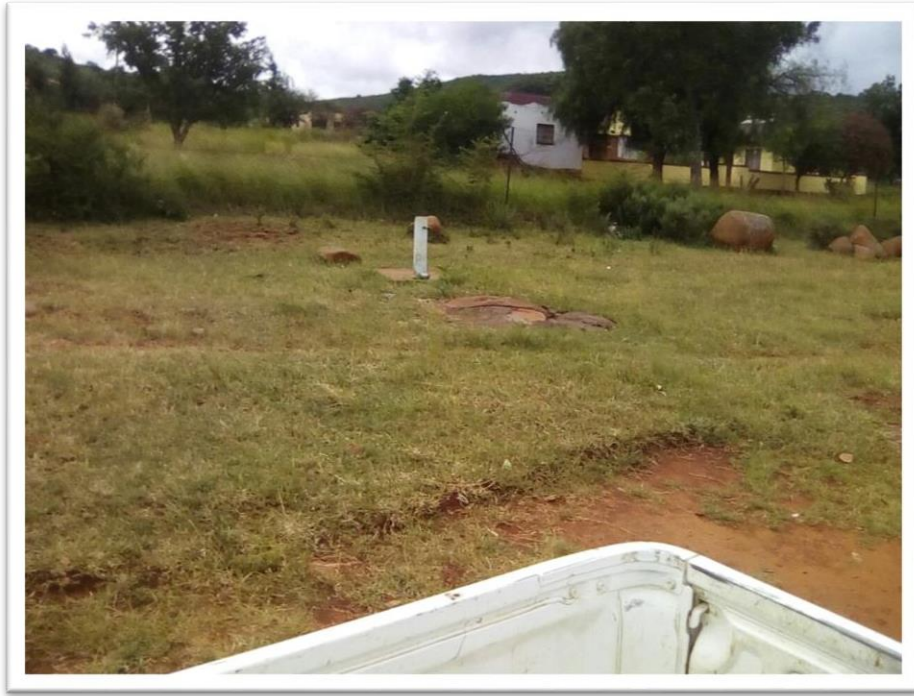
Figure 15: Damaged Water Infrastructure at Kampeng Section
