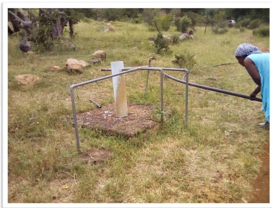
Figure 18: Interconnections and Illegal Water Connections at Kampeng Section
