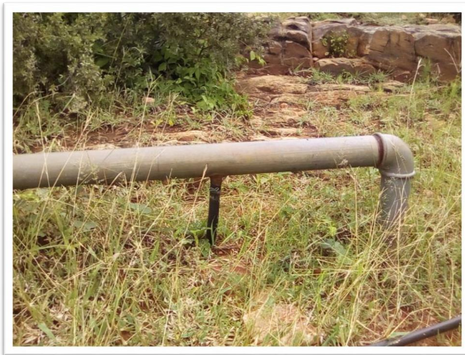
Figure 16: Illegal Connection on a steel pipe at Kampeng Section
